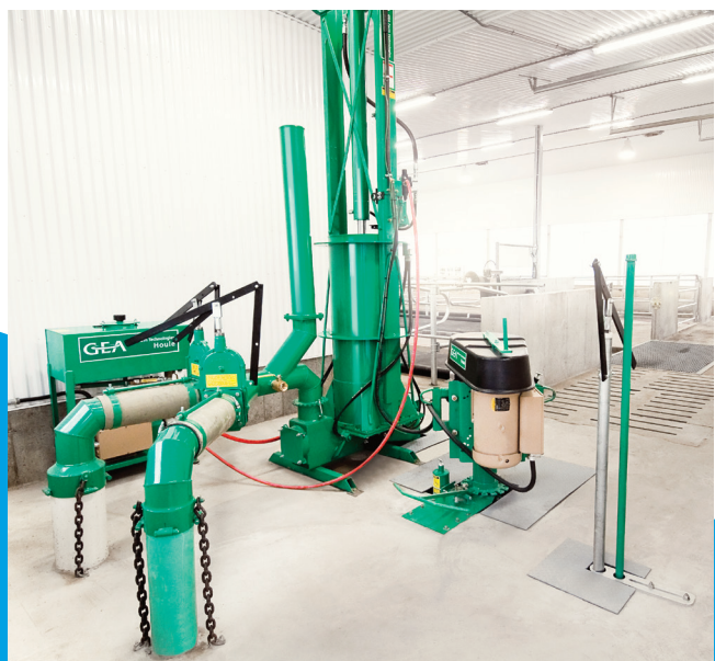
Electromix system on the floor above the reception pit. Installation with double discharge for manure transfer in two different pits.
